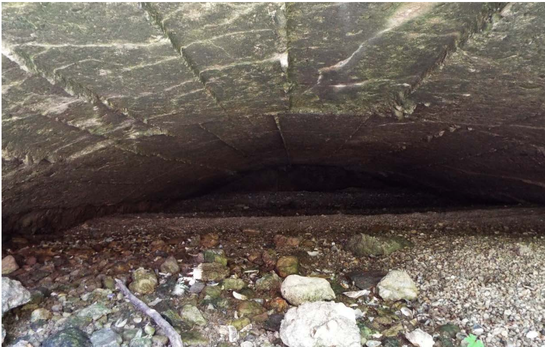
This pre-1897 flume on the west side, usually under water, is almost filled with silt.
